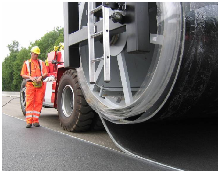
Figure 5: The operator controls the movement of the asphaltmat and places it very precisely.
