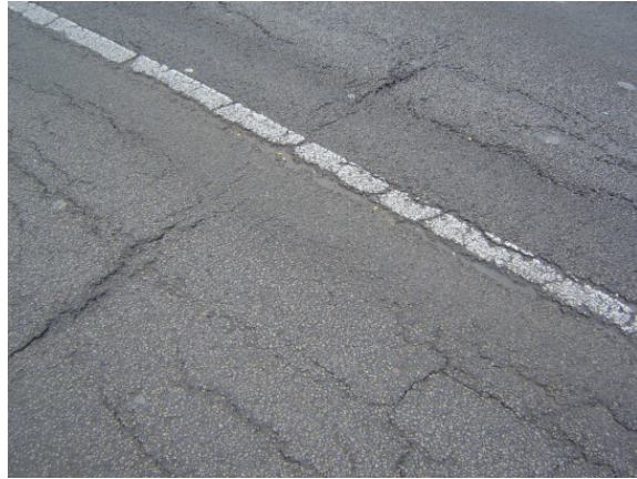
Figure 2: Cracks in Mastic Asphalt layer
