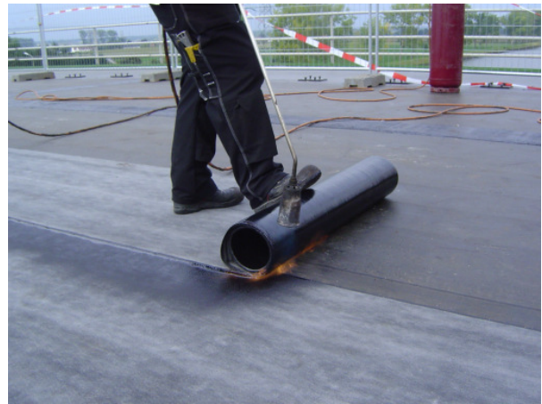
Figure 5: Melting the membrane
